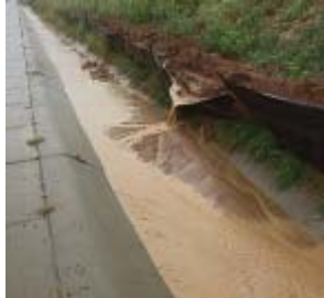
Sediment from construction site
