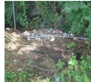
Trash/debris from construction site
